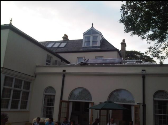
'Grange Hall', Guernsey – Very Large & Very Leaky
